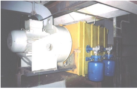
PRAF CARBUNE Celula desprafuire CENTRALA TERMOELECTRICA BRASOV-ROMANIA
