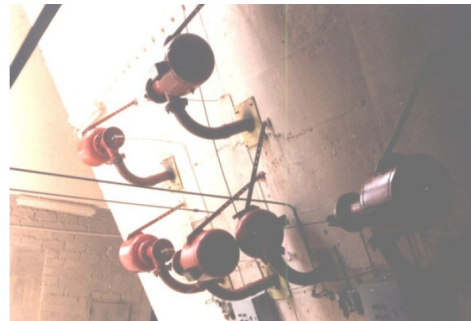
RAW STOCK FOR CEMENT Concrete silo LAFARGE ROMCIM SA HOGHIZ-ROMANIA
